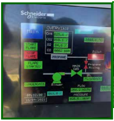
Control panel of flare operating
