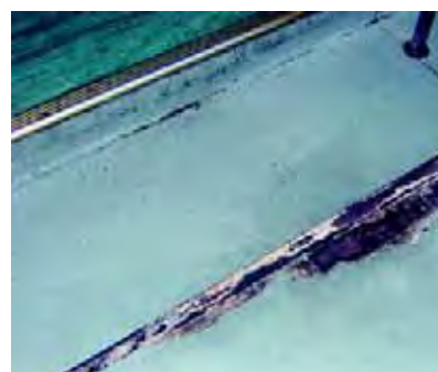
Defective flooring requiring attention
