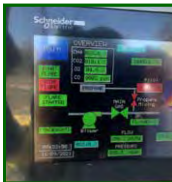
Control panel of flare operating
