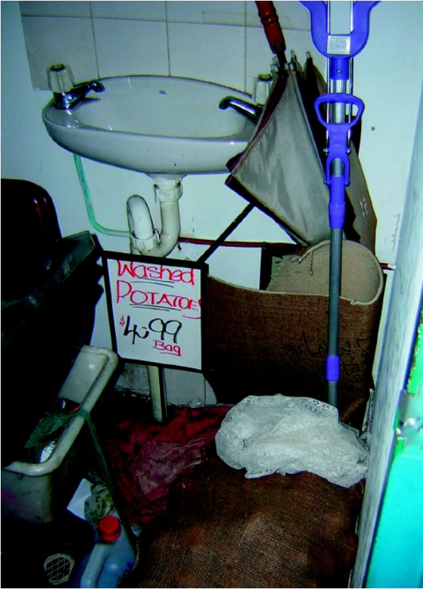
Obstruction of hand wash basin
