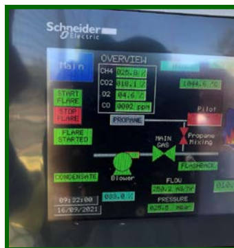
Control panel of flare operating
