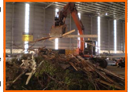
Resource recovery within the Facility
