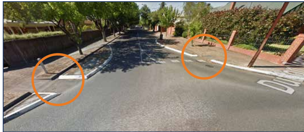
Pedestrian ramps do not align
